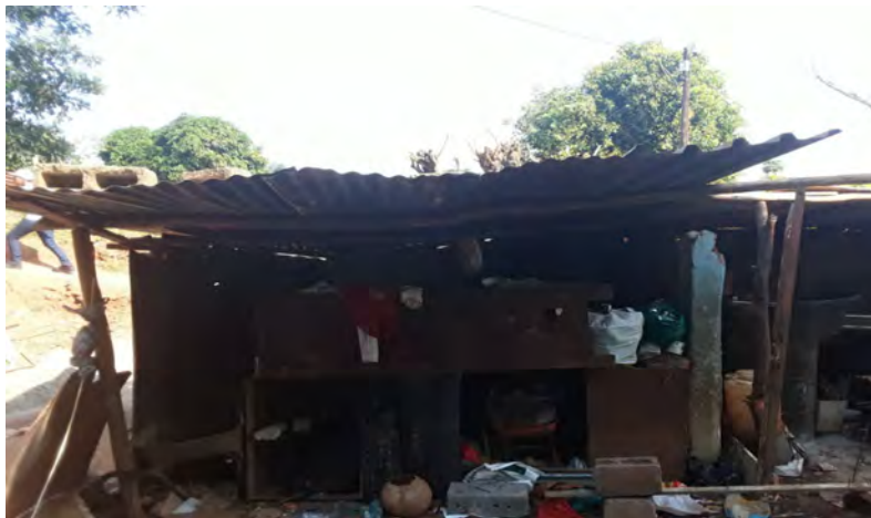
Figure : Conveys the aftermath following a heavy rainfall incident in Lloyd (Ward 14)
