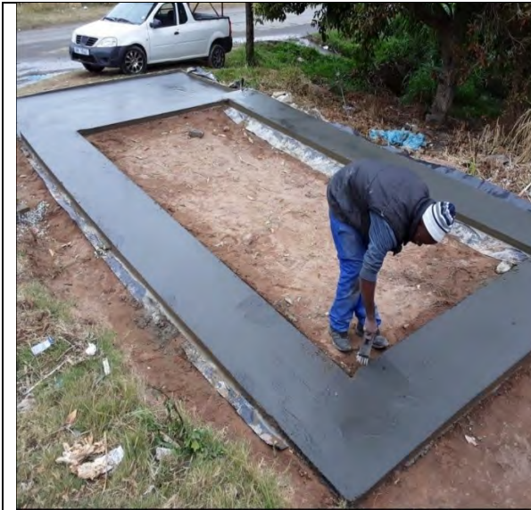
Slab completed for the container to be installed at Ward 18 for Siyanda Mfeka
