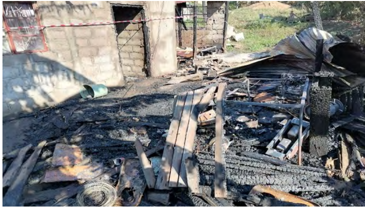
Figure : A house damaged by structural fire in Ward 29, Charlotteddale.
