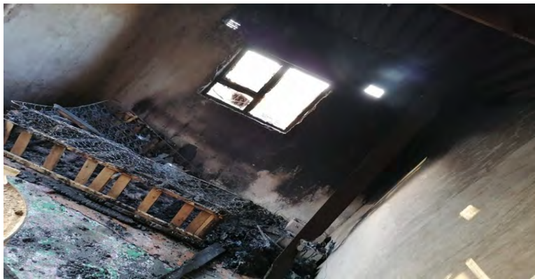
Figure : A house damaged by structural fire in Ward 7, HSE No 140
