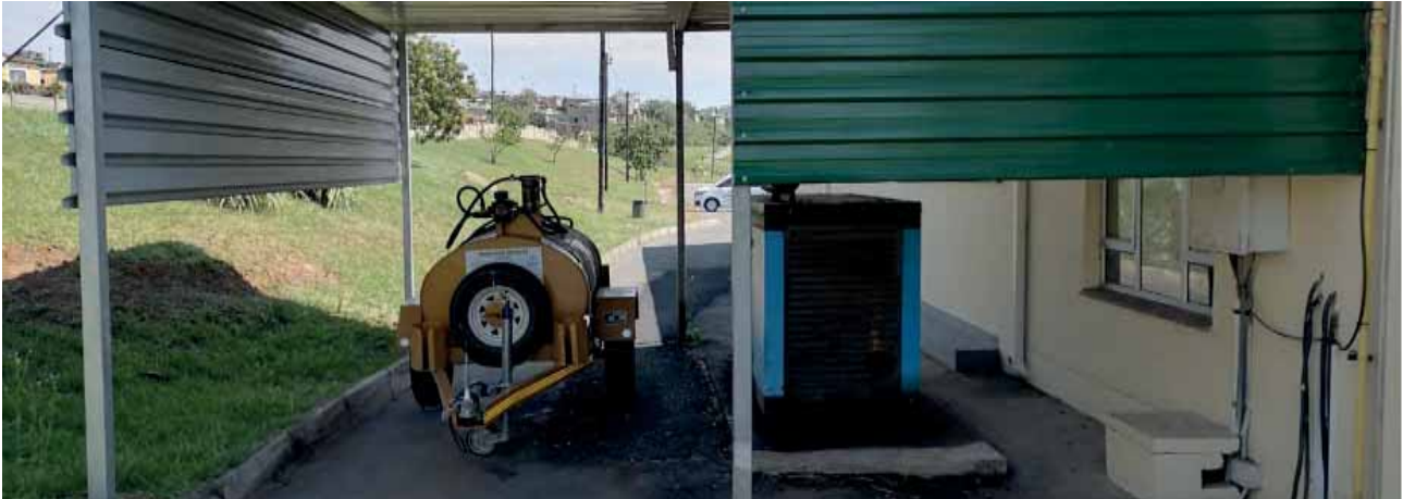
Extended Shelter for the Backup Generator and The Diesel Tank
