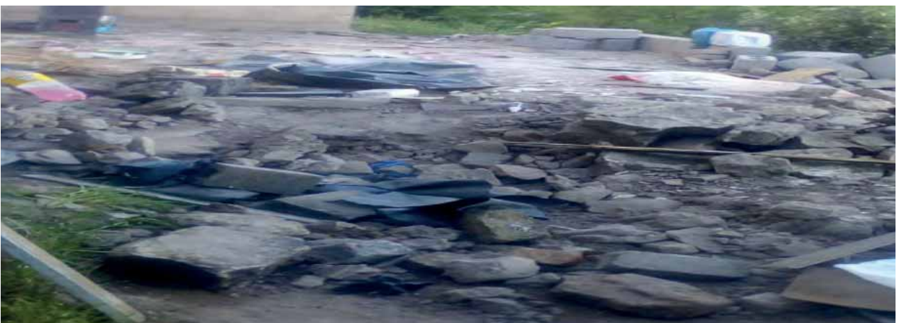
Figure 09: Conveys the aftermath following a heavy rainfall incident in Ward 17 (Monkey Town)
