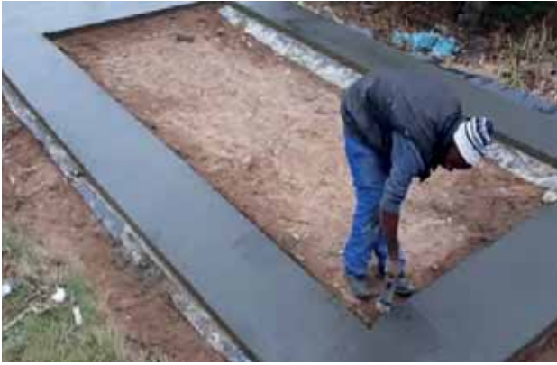
Slab Completed for the Container to be Installed at Ward 18 for Siyanda Mfeka
