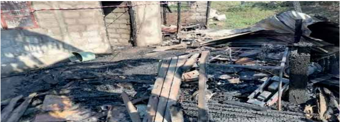
Figure 10: A house damaged by structural fire in Ward 29, Charlotteddale
