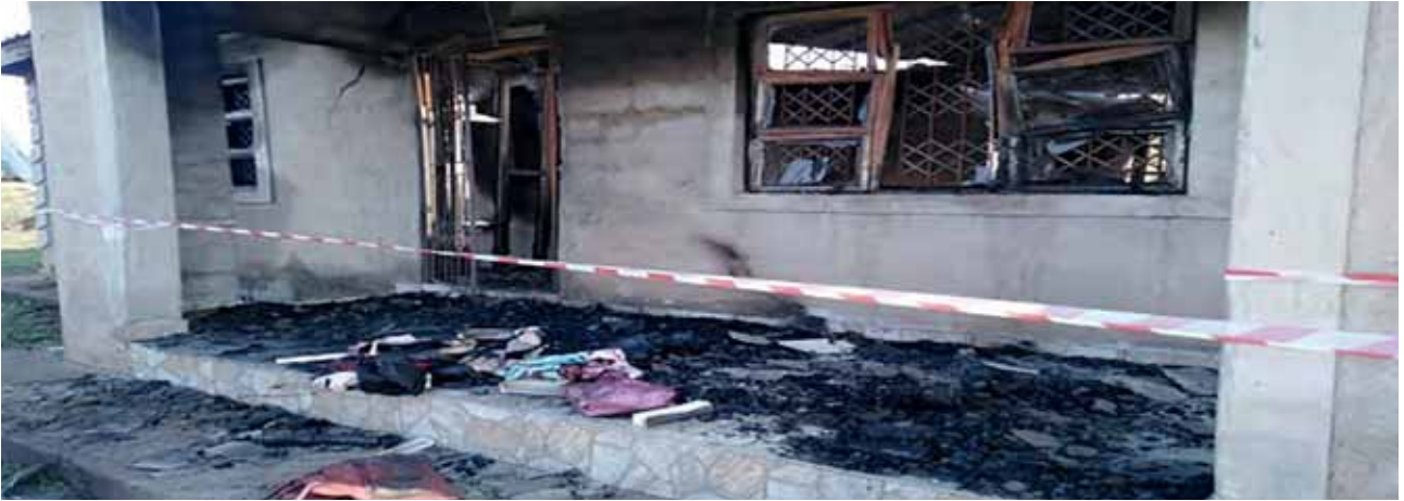
Figure 07: Conveys the aftermath following the structural fire incident that resulted in one fatality in August 2020 in Ward 26, Ntshawini area.
