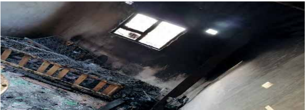
Figure 11: A house damaged by structural fire in Ward 7, HSE No 140
