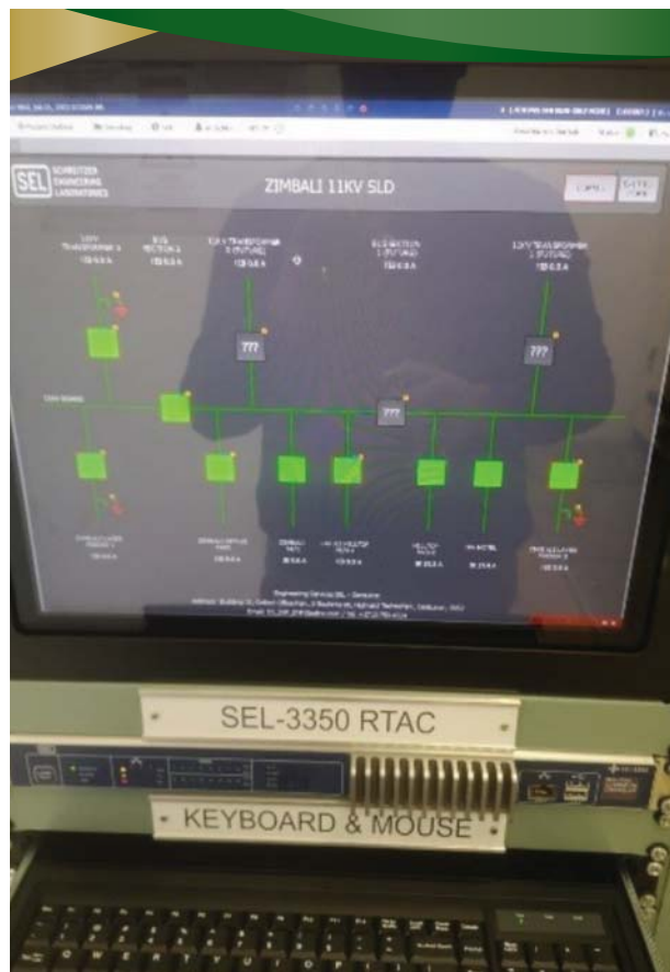
SCADA HMI screen at Zimbali substation
