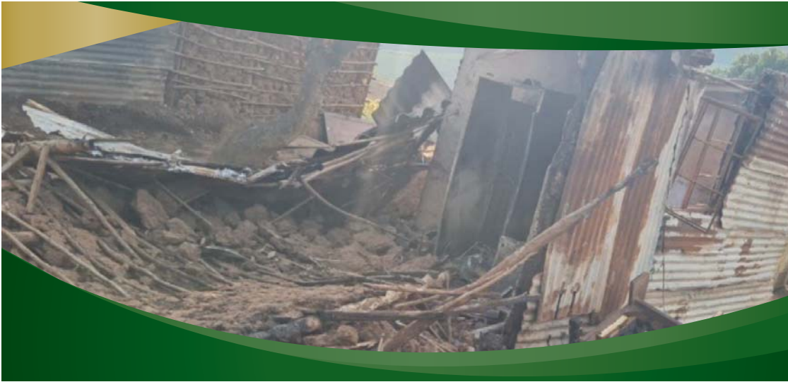
Aftermath following a heavy rainfall incident in Ward 15 (Chris Hani) during the month of September 2022
