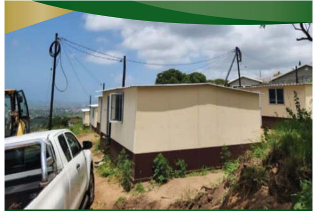
Temporary Residential Units (TRU's) electrified.
