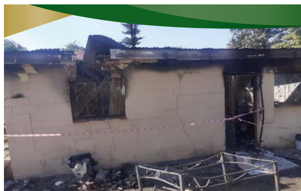
Aftermath following a Heavy Rainfall incident in Ward 9 (Cranbrook) during the month of June 2023
