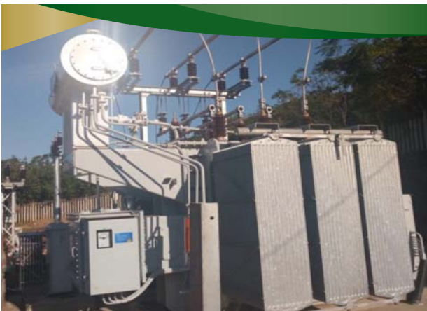
Zimbali Substation new transformer
