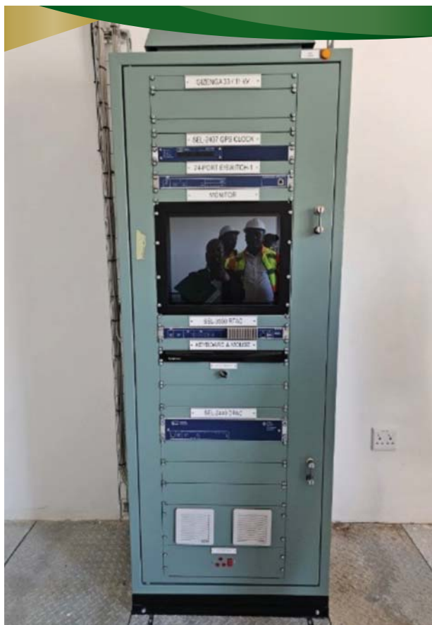
SCADA panel in Gizenga substation
